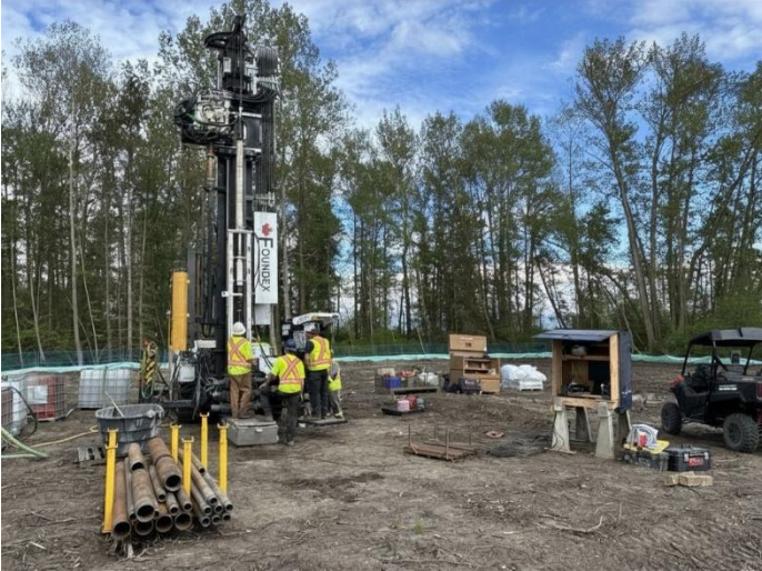
Figure 2: Drilling equipment on the Deas Island Project site – as part of Geotechnical investigations to support the design of tunnel elements.
