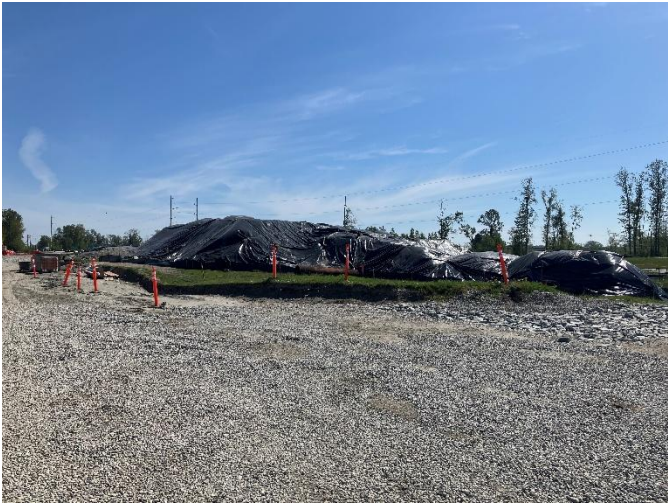
Figure 3: Preload on the Deas Island Project site for use in improving ground stability.
