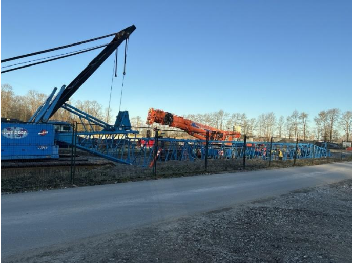
Figure 1: Demobilization of crane used for onshore piling works testing on the Deas Island Project site.
