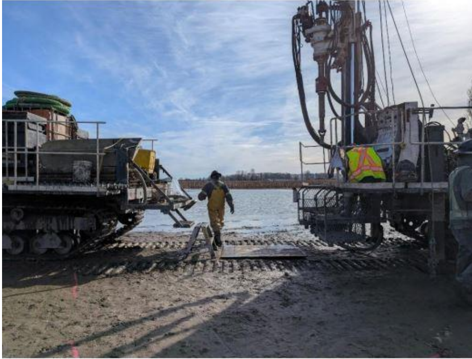
Figure 1: Preparing the drill rig for onshore geotechnical investigations near the Richmond Bike Shuttle.
