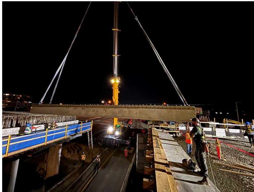
Image 3: A heavy-lift crane hoisting an end-span girder into position between the main-span girders and the northeast abutment.
