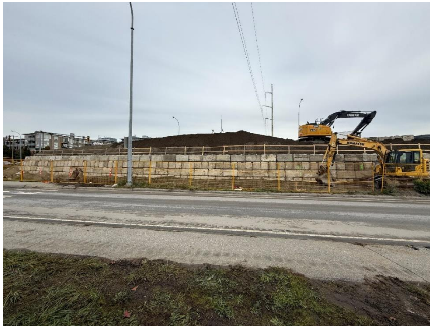
Figure 3: Preload placement in the southwest quadrant, with a temporary retaining wall in place.
