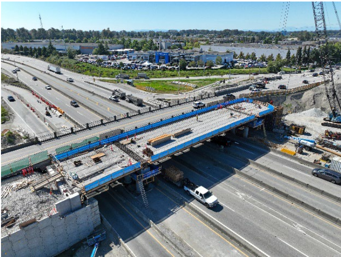
Image 2: Drone image facing southwest showing all Phase 1 girders in place and deck construction
