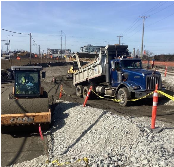
Crews re-aligning the on-ramp between Steveston Highway and Highway 99 northbound in March 2023.
